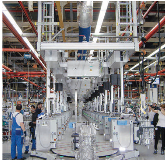
Overhead structure built from Series 40 profiles to support supply lines for assembly workstations
