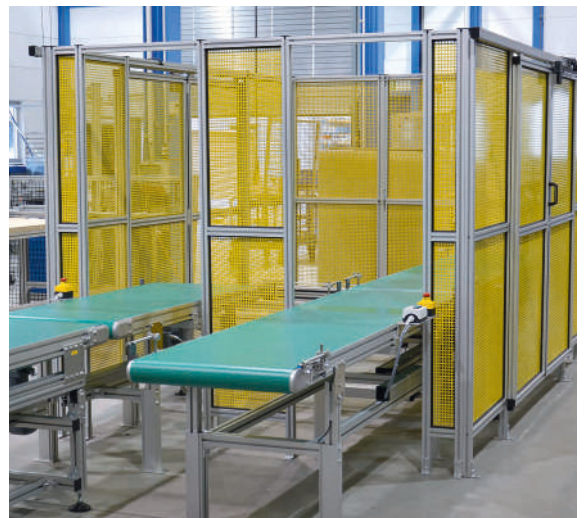
Custom protective device guard made from partitions with powder-coated perforated sheets and sliding doors with solenoid latches
