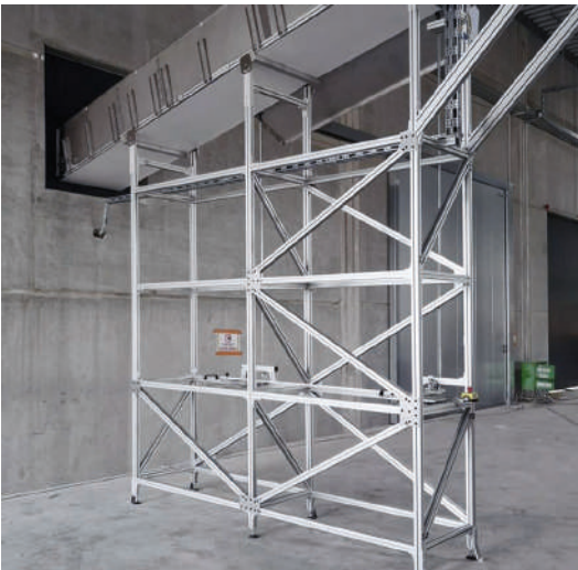
Frame and suspension for conveying path at a height of 5 m below the hall ceiling
